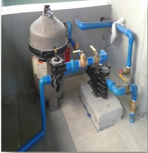
e Swimming Pool Pumps and Drain Line
