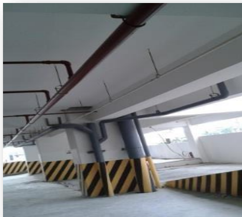
g Fire Protection, ITC and Auxiliary Drain Line
