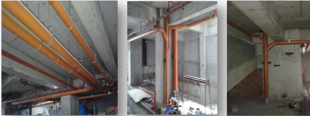
b Parking Drain Line
